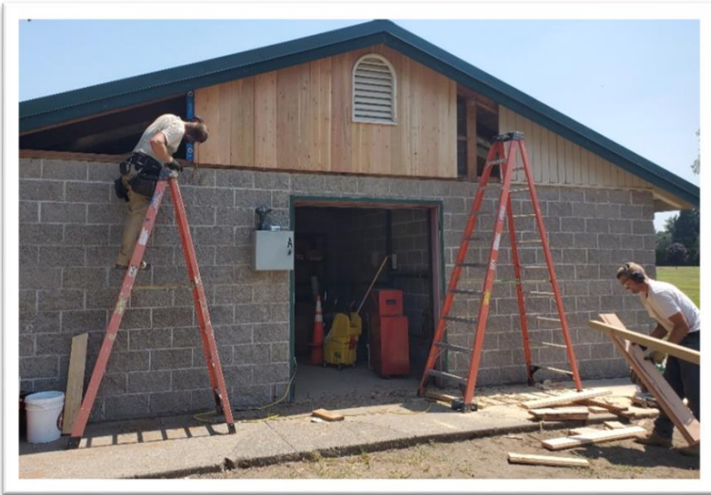
Volunteer group from SDA replaced rotted wood on the upper portion of the bathroom at Meldrum Bar Park.
