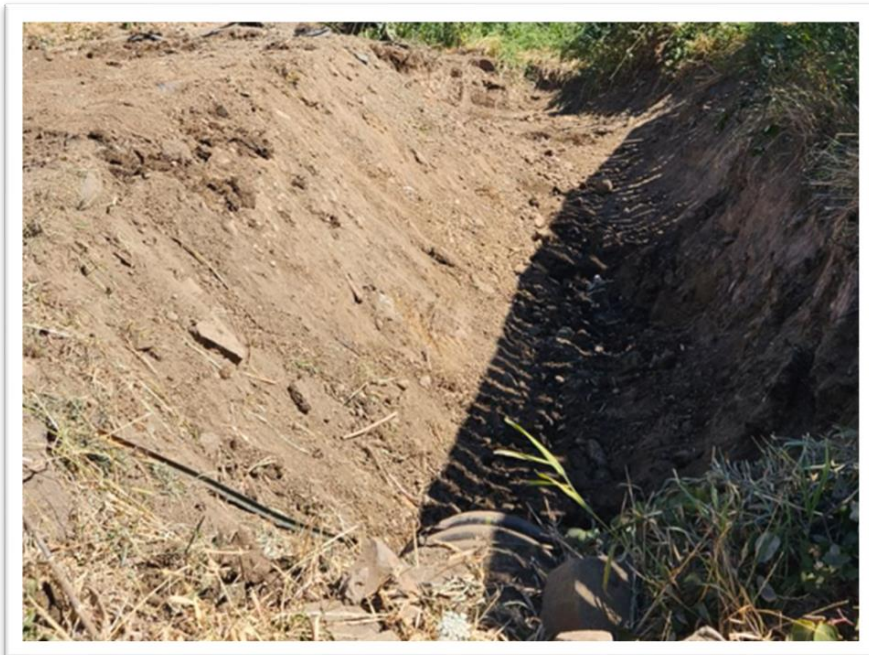
Dugout the ditch coming from Glen Echo which floods the road, below
