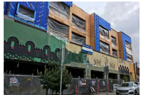
A former single-story automobile repair shop being redeveloped with additional stories for residential (Alberta neighborhood, Portland, OR)
