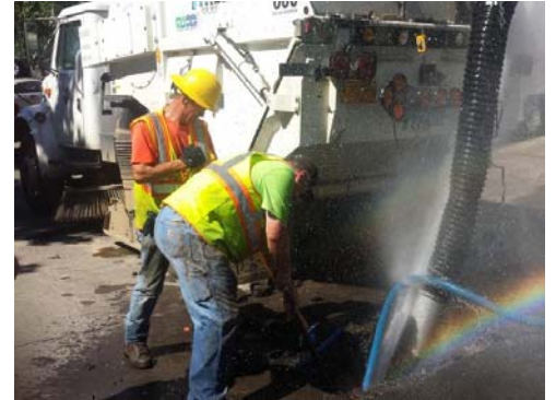
Public Works crews repair a water pipe blowout—one of more than 34 since May 2016. Implementing a pipe replacement program will greatly reduce service interruptions for our customers.
