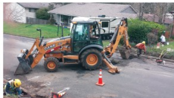
City crews on the scene replacing a leaking water pipeline. An aging line had been repaired three times in the past and needed to be replaced.
