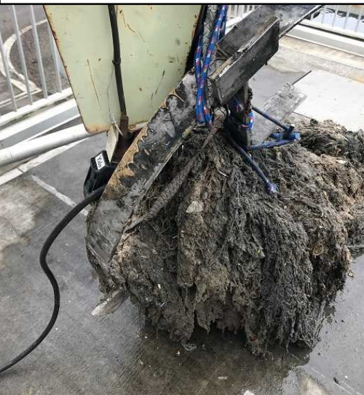
Below photo from Pamplin Media Group: Sewer blockage removed by Oak Lodge Water Services District on Tuesday, January 26, 2021 caused by flushed paper towels, wipes and rags.
