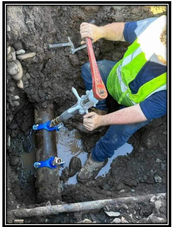
Crewmember Eric Fanning using the tapping machine to re-tap the water main for the new service lines on Portland Ave. (Pictured right)
