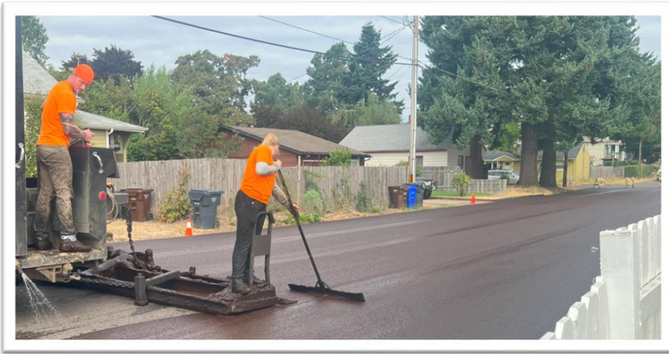
The Annual Slurry Seal Project, crews from Blackline, Inc. work to apply the slurry seal emulsion on Barton Ave.
